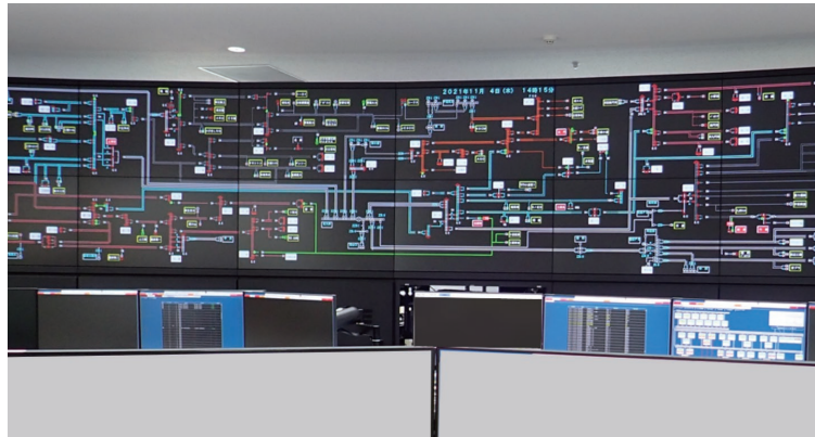
Renovated control room at Kitakyushu Branch Office of Kyushu Electric Power Transmission and Distribution Co., Inc.
