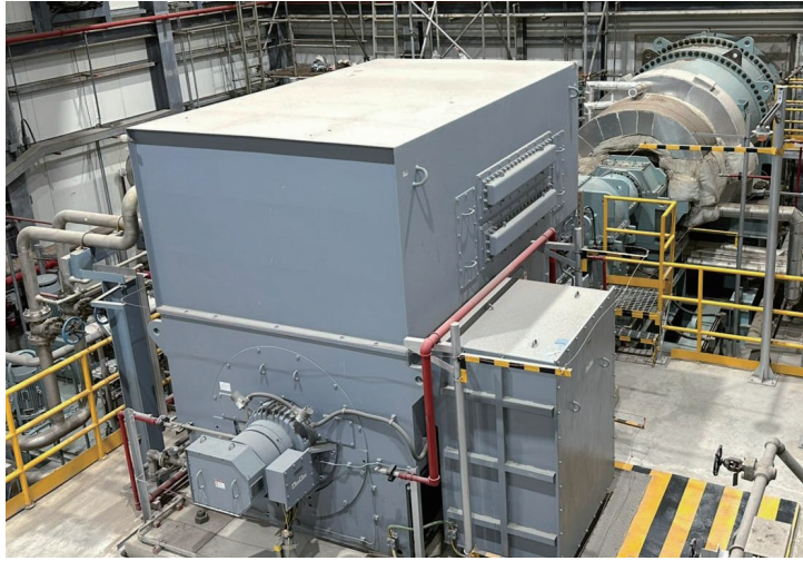
Tanawon Geothermal Power Plant steam turbine generator
