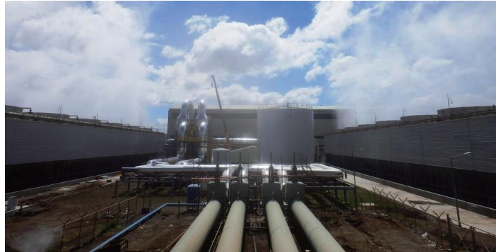
Olkaria I Geothermal Power Plant
