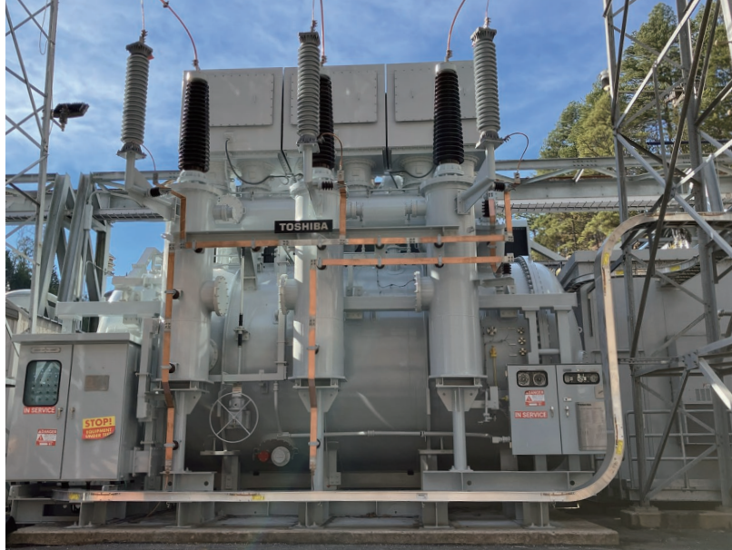
138 kV–300 MVA GIT commencing commercial operation
