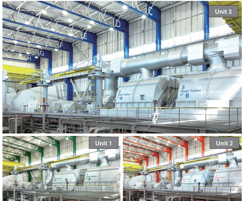
Steam turbine and generator
