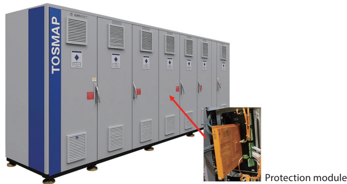
Turbine control panel
