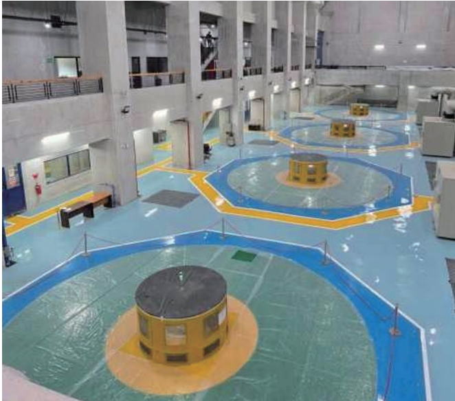
Equipment layout inside Kerinci Merangin Hydroelectric Power Plant (PLTA Merangin) building
