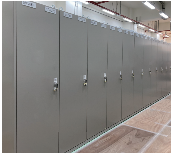
New control and relay panel for Taiwan High Speed Rail
