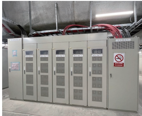
TESS Installed at Line 6 substations
