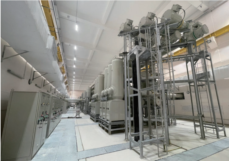
400 kV GIS at New Babil 400 kV Substation, Iraq
