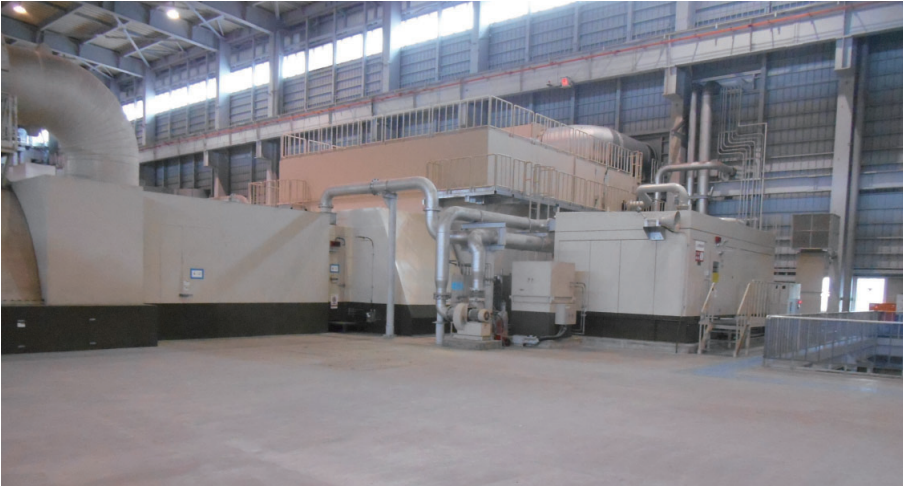
Updated gas turbine enclosure and fuel gas skid at JERA Co., Inc. Futtsu Thermal Power Station Unit 4-2
