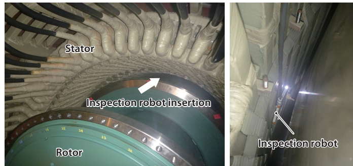
Detailed inspection of turbine generator applying inspection robot at Barakah Nuclear Energy Plant Unit 1, United Arab Emirates
