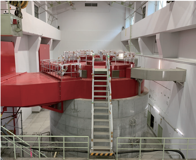
Hydraulic turbine generators at the Chubu Electric Power Co., Inc. Kuze Hydroelectric Power Station
