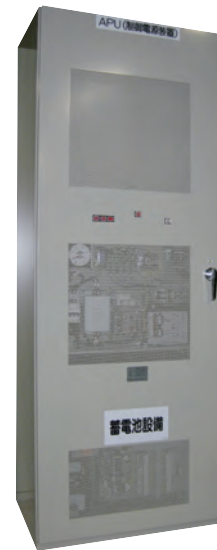
Auxiliary power unit
