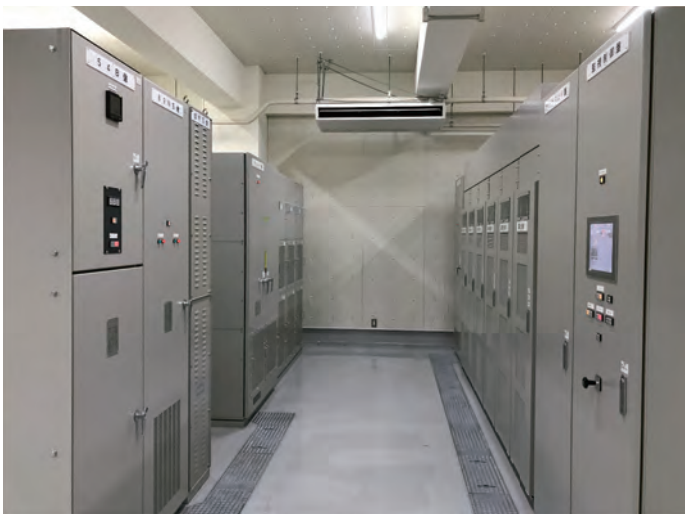
Traction energy storage system of Okinawa Urban Monorail, Inc.
