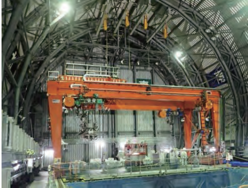
Fuel handling machine installed at Fukushima Daiichi Nuclear Power Station Unit 3
