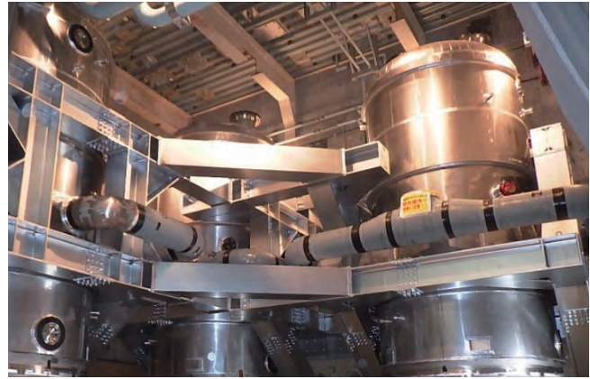
FCVS after installation
