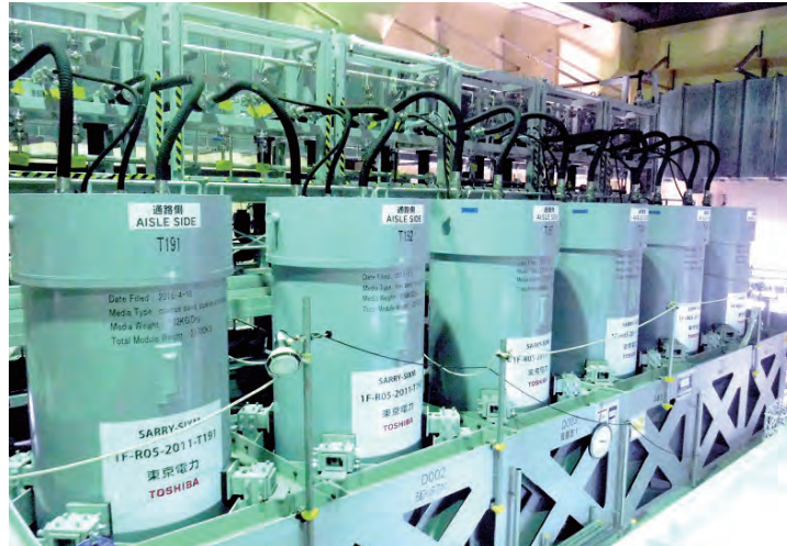
Two filtration filters and four adsorption towers of SARRY II
