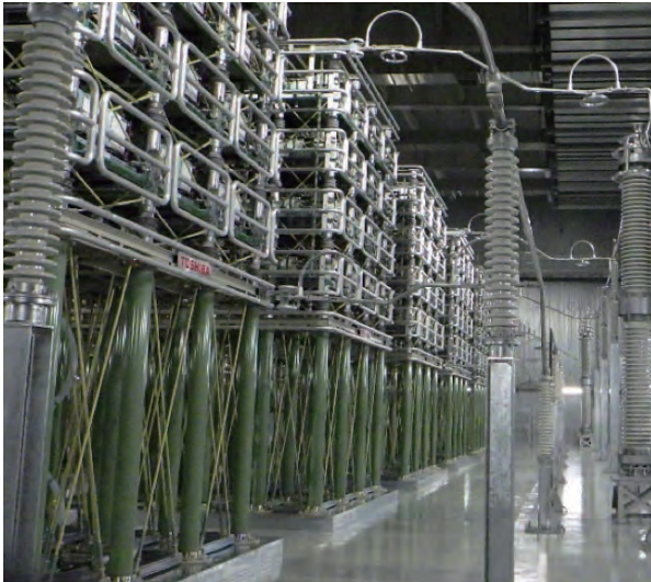
Voltage-source converters for New Hokkaido-Honshu HVDC Link
