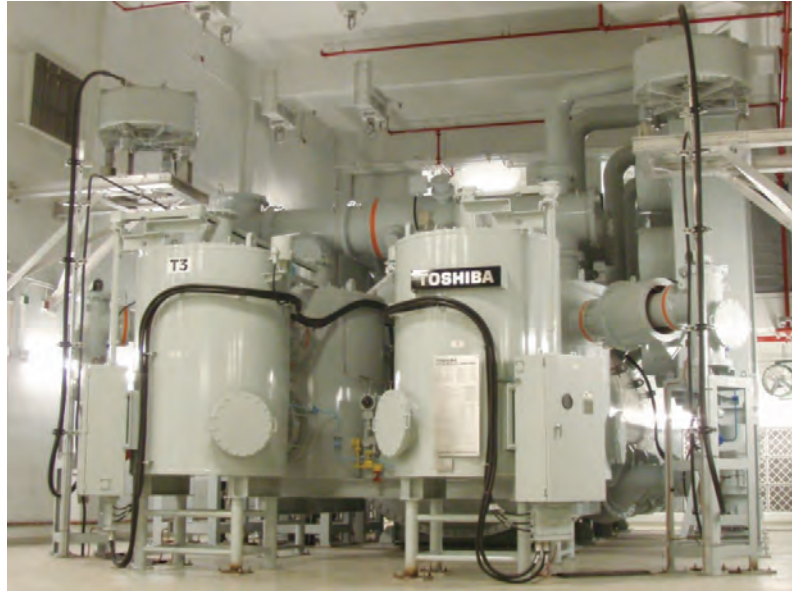
GITs installed at underground substation of Toronto Hydro-Electric System Ltd., Canada
