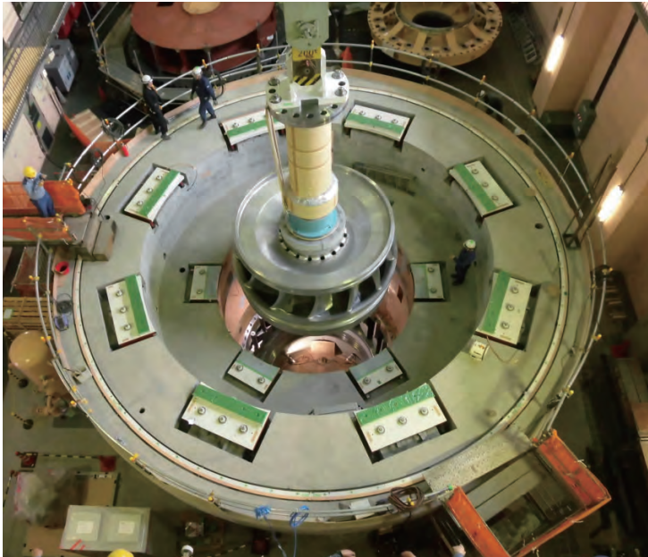
Installation of hydraulic runner at Maruyama Power Station Unit 2 of The Kansai Electric Power Co., Inc.
