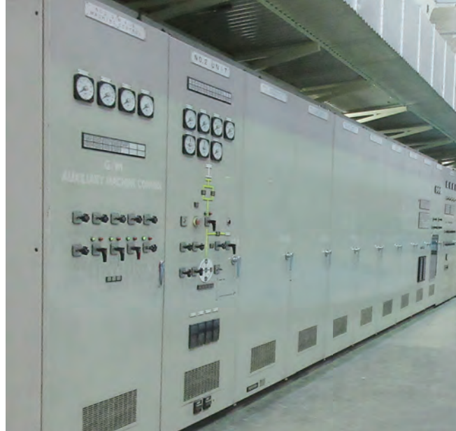
Partially renewed main control board
