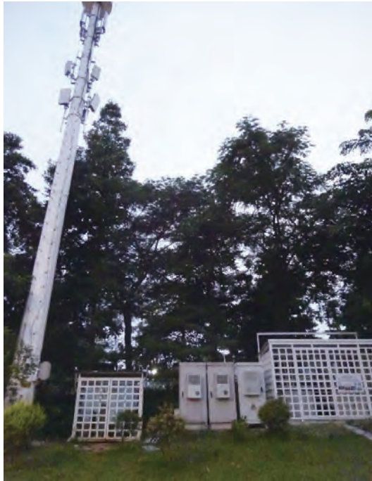
Base station for 5G mobile communications in Guangzhou, China
