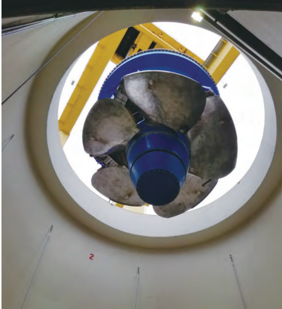
Installation of third Kaplan turbine runner at Wells Hydroelectric Power Plant, U.S.A.
