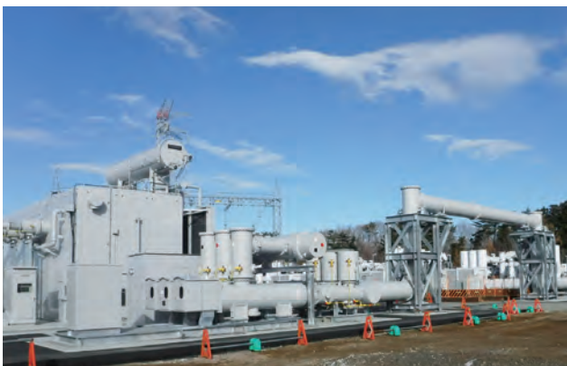
都路変電所に設置した500 kV 変電設備 500 kV substation facilities installed at Miyakoji Substation of Fukushima Power Transmission Co., Ltd.
