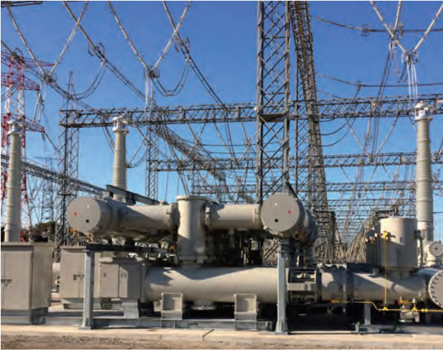
新佐原変電所に設置した550 kV GIS 550 kV GIS installed at Shin-Sawara Substation of TEPCO Power Grid, Inc.
