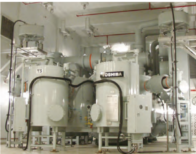
地下変電所に設置したGIT Gas-insulated transformers (GITs) installed at underground substation of Toronto Hydro-Electric System Ltd., Canada
