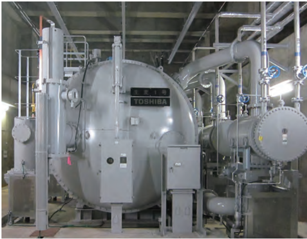
墨東変電所 300 MVA GIT 300 MVA GIT installed at Bokuto Substation of TEPCO Power Grid, Inc.
