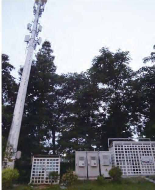
中国広州市の5G通信基地局 Base station for fifth-generation (5G) mobile communications in Guangzhou, China
