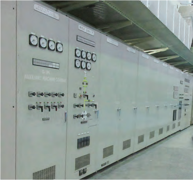
部分更新を行った主配電盤 Partially renewed main control board for River Bed Pumped Storage Power Station, India
