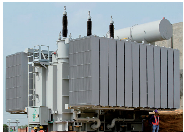
Scott connected transformer installed on-site in dedicated freight corridor, India
