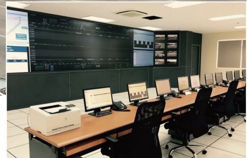
Traffic control center
