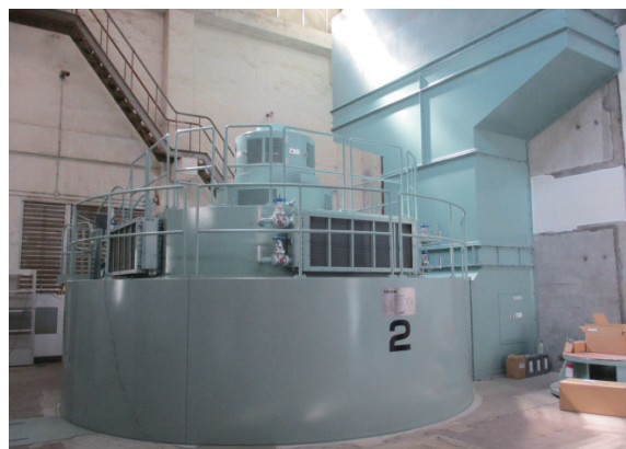
Hydraulic turbine generator
