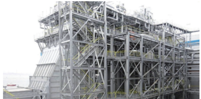
Overall view of heat recovery steam generator
