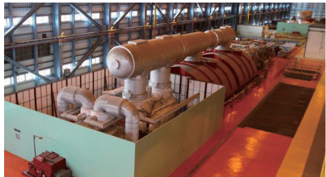
Steam turbine generator
