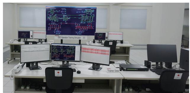
Substation operation training simulator
