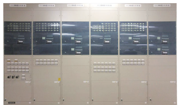
Control equipment (digital protective relays)
