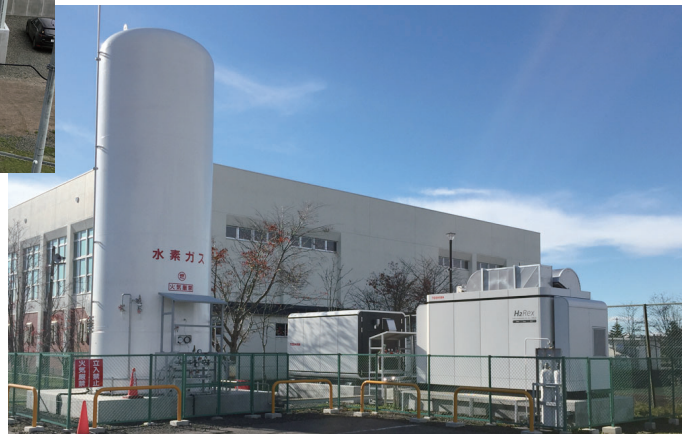
Hydrogen application facility installed at heated pool
