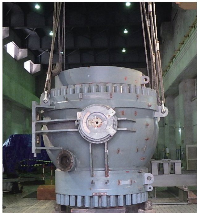
View of inlet valve during overhaul of Bakaru Hydro Power Plant Unit 1
