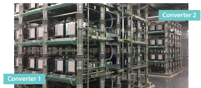
VSCs used in demonstration tests
