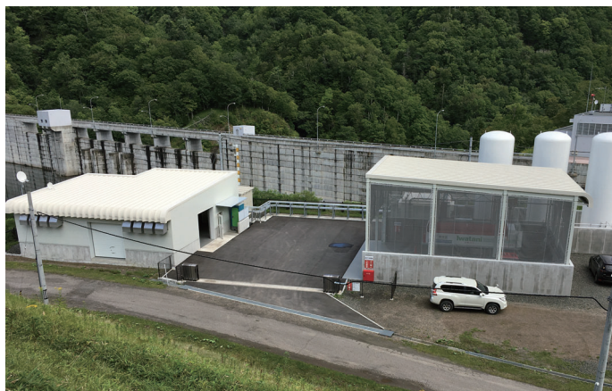
Hydrogen production facility installed at Shoro Dam in Hokkaido, Japan
