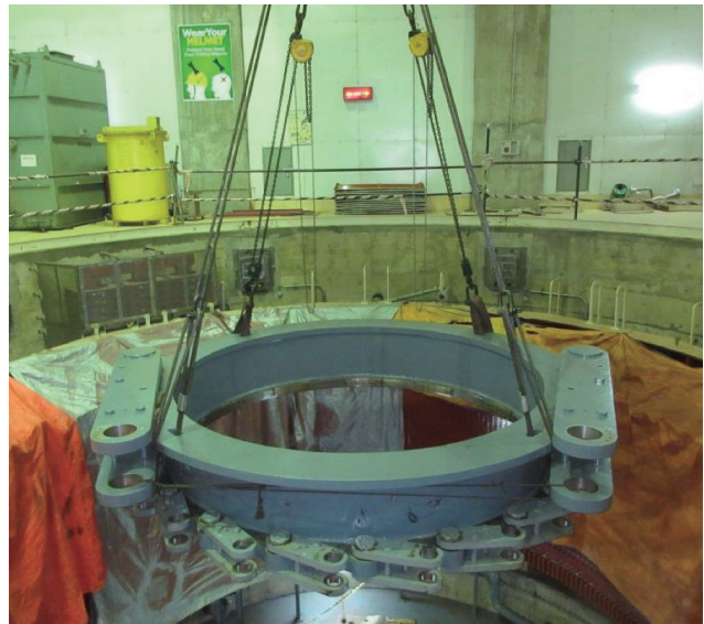
Installation of turbine guide ring during overhaul of Purulia Pumped Storage Power Station Unit 1
