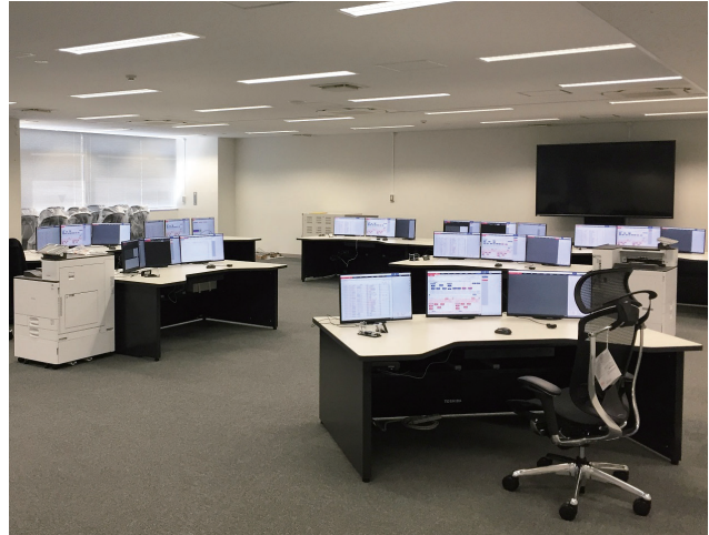
Central SCADA system for hydroelectric power stations of TEPCO Holdings, Inc.
