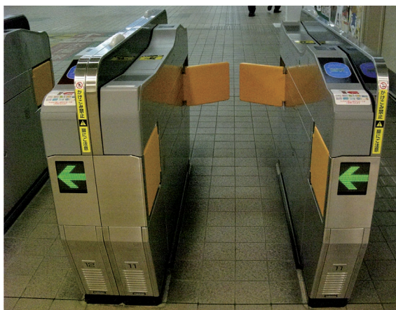
IC 専用自動改札機 Standard automatic ticket gate for dedicated integrated circuit (IC) card use
