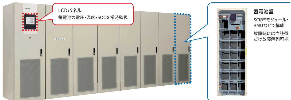
UPS用 SCiB™蓄電システム SCiB™ lithium-ion rechargeable battery energy storage system for uninterruptible power systems (UPS)
