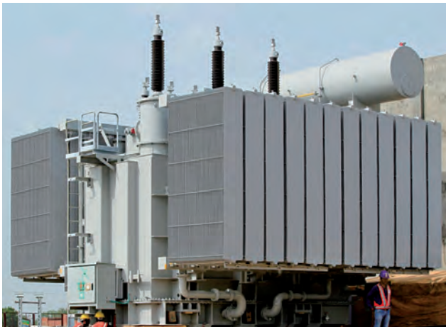
現地に据え付けられたスコット変圧器 Scott connected transformer installed on-site in dedicated freight corridor, India
