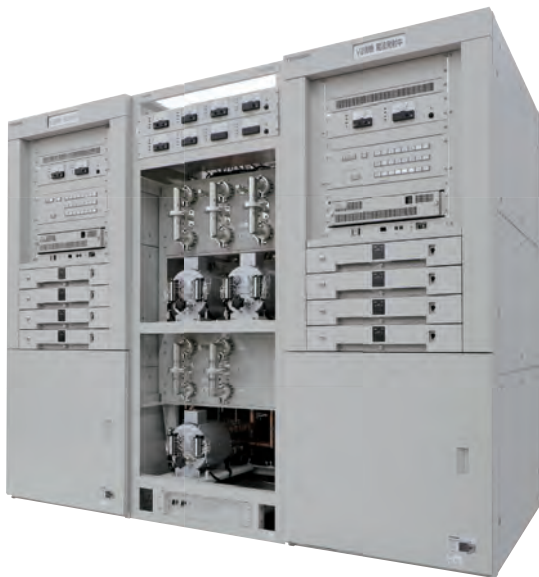
東京 芝放送所 1 kW 実験試験局用送信設備 1 kW transmitter for advanced digital terrestrial TV broadcasting installed at Shiba experimental station of Japan Broadcasting Corp.
