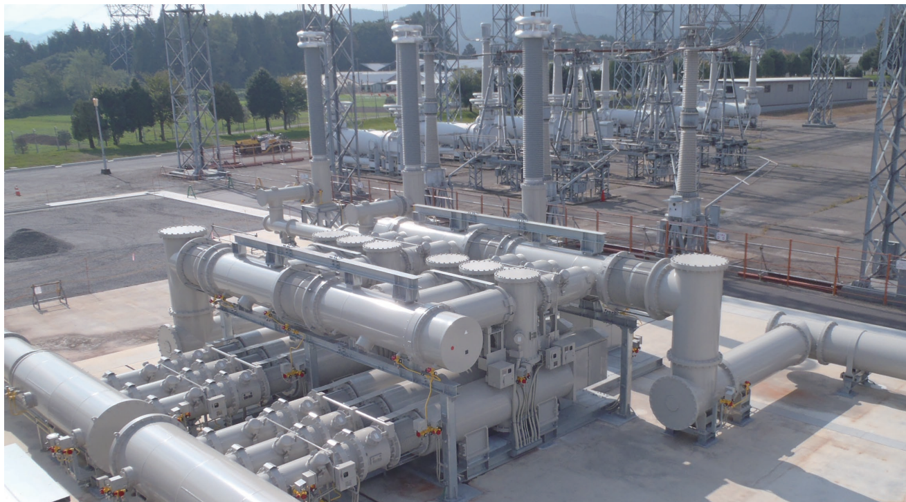
新信濃変電所 550 kV ガス絶縁開閉装置 550 kV gas-insulated switchgear for Shin-Shinano Substation of TEPCO Power Grid, Inc.
