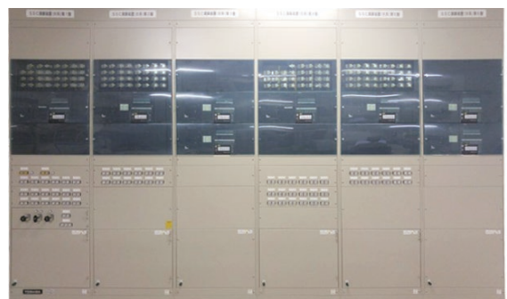
演算装置 (デジタルリレー) Control equipment (digital protective relays)
