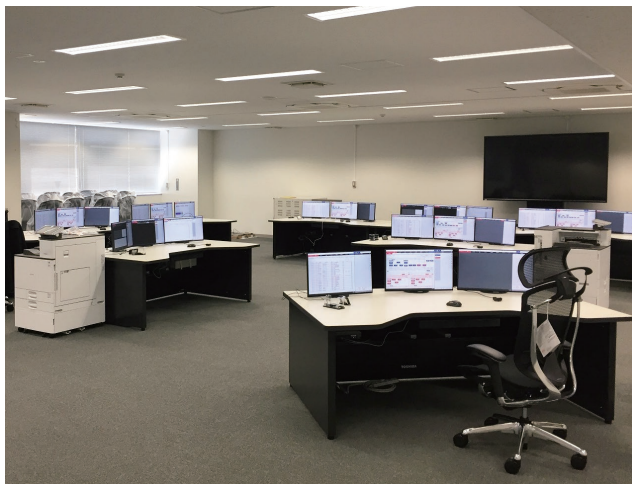
水力発電所集中監視制御装置 Central supervisory control and data acquisition (SCADA) system for hydro-electric power stations of Tokyo Electric Power Company Holdings, Inc.
