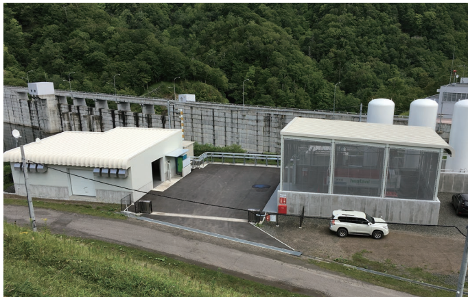
庶路ダムに設置した水素製造施設 Hydrogen production facility installed at Shoro Dam in Hokkaido, Japan
