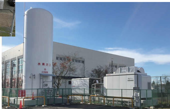
温水プールに設置した水素活用機器 Hydrogen application facility installed at heated pool
