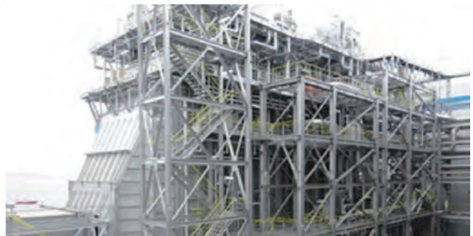
HRSG全景 Overall view of completed heat recovery steam generator (HRSG)
