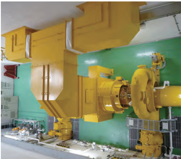
横軸二輪単流両掛けフランシス水車及び発電機 Horizontal-shaft, two-runner, single-discharge, double-spiral Francis turbine and generator for Sakashu Power Plant in Tokushima, Japan
