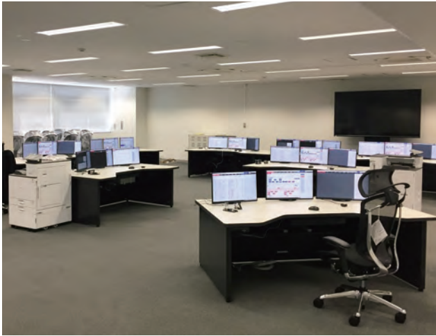
水力発電所集中監視制御装置 Central supervisory control and data acquisition (SCADA) system for hydro-electric power stations of Tokyo Electric Power Company Holdings, Inc.
