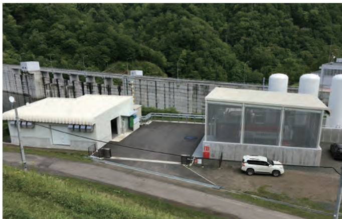
庶路ダムに設置した水素製造施設 Hydrogen production facility installed at Shoro Dam in Hokkaido, Japan
