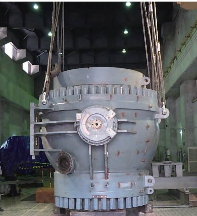
入口弁オーバーホール時の様子 View of inlet valve during overhaul of Bakaru Hydropower Plant Unit 1, Indonesia
