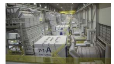
Gas turbine and generator
