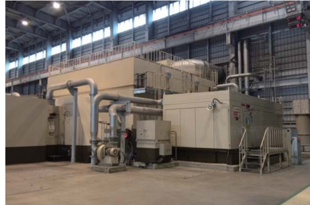
Renewed gas turbine enclosure and fuel gas skid at Futtsu Thermal Power Station Unit 4-1 of TEPCO Fuel & Power, Inc.
