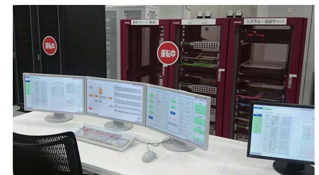
Processing equipment of trunk transmission ISC system of Chubu Electric Power Co., Inc.
