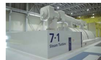
Steam turbine and generator
