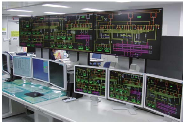
Distribution control system of TEPCO Power Grid, Inc.
