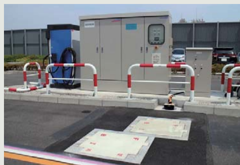
Transmitting equipment of 44 kW rapid wireless charging system
