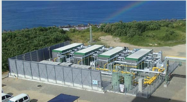
Biogas cogeneration plant at Ginowan Sewage Treatment Center
