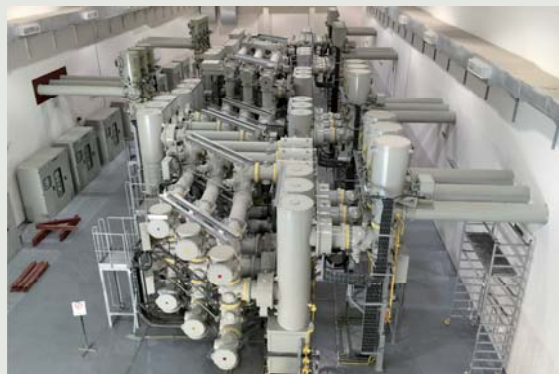
400 kV GIS for Jahloot Grid Station, Oman
