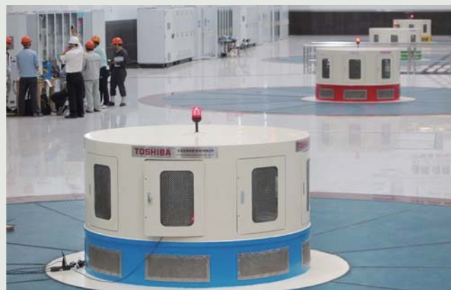
Immediately before load rejection, with red operation lamps on all four units illuminated
