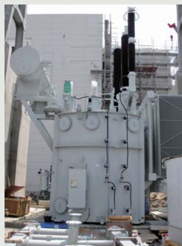
333.3 MVA-525 kV transformer for Chaeng Wattana Substation, Thailand
