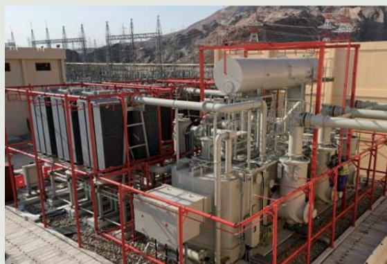
500 MVA transformer for Jahloot Grid Station
