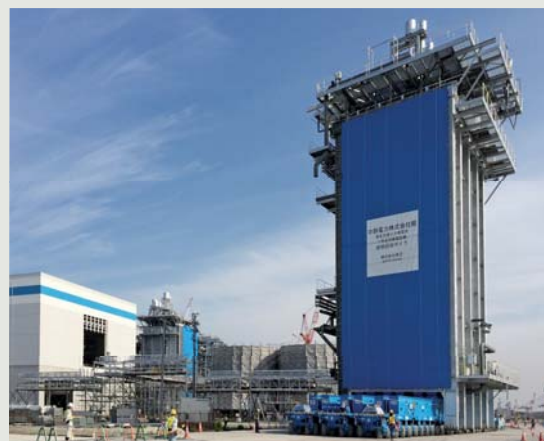
7-1(A) HRSG for Nishi-Nagoya Thermal Power Station Group No. 7 of Chubu Electric Power Co., Inc.
