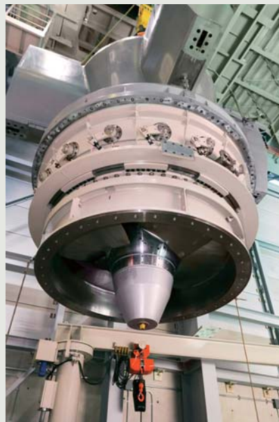
Installation of water turbine at Daini Yabukami Hydroelectric Power Station of Tohoku Electric Power Co., Inc.
