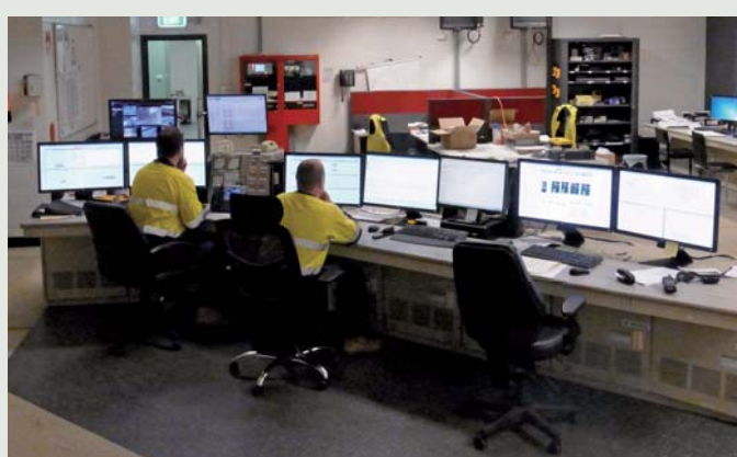
Upgraded operator station in central control room of Tarong North Power Station, Australia
