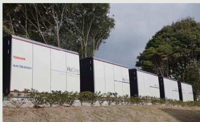
H 2 One™ hydrogen-based autonomous energy supply system installed in West Arm of Henn na Hotel Huis Ten Bosch
