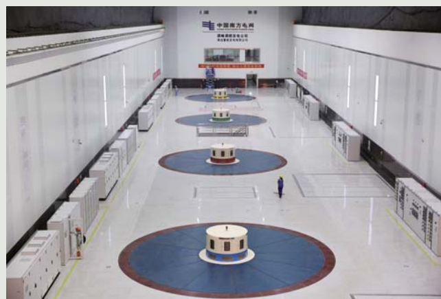
Qingyuan Pumped Storage Power Station, China
