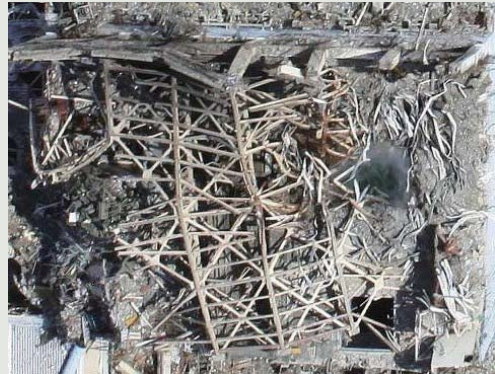
Operating floor of Fukushima Daiichi Nuclear Power Station Unit 3 covered with collapsed building frames after Great East Japan Earthquake (before removal of large debris)
