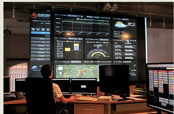
VPP control center of Elektro Ljubljana d.d.
