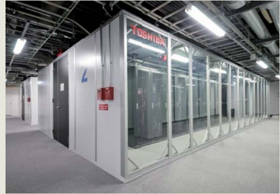
Toshiba Indoor Modular Data Center
