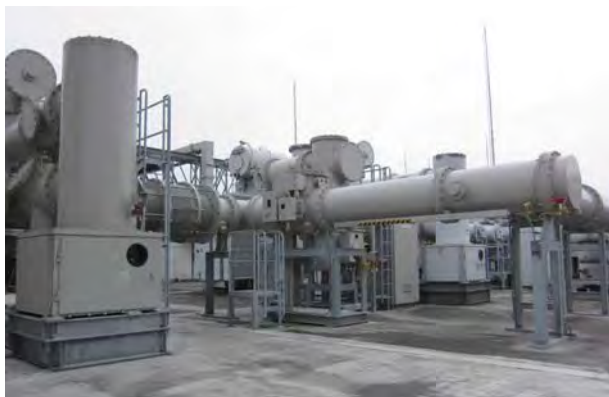
埼玉県中川流域下水道終末処理場 特別高圧4号バンク設備 No. 4 extra-high-voltage power receiving equipment installed at Nakagawa River Basin Sewage Disposal Plant, Saitama
