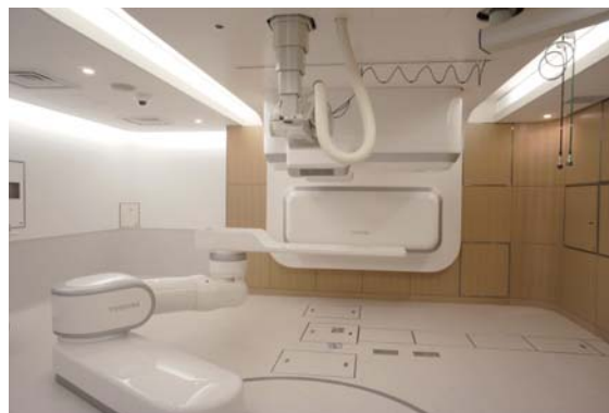
Heavy ion treatment room for irradiation system
