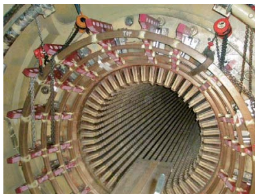
Generator stator coil of Lambton Generating Station, Canada
