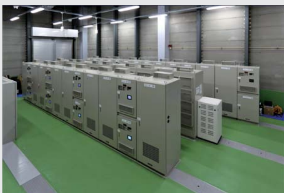
▲ SCiB™を用いた蓄電池システム Storage Battery System using SCiB™ rechargeable batteries
