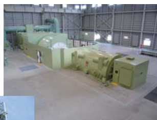
Power train of Unit 4
