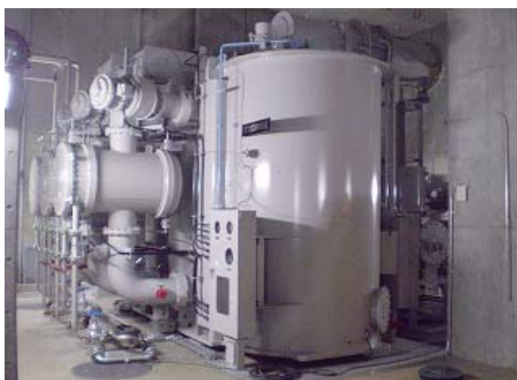
60 MVA-66 kV ガス絶縁変圧器 60 MVA-66 kV gas-insulated transformer (GIT)
