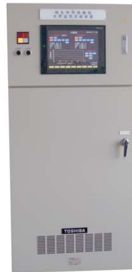
Demonstration unit of water quality monitoring support system
