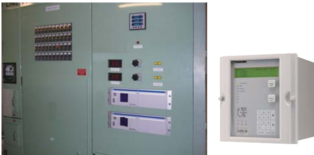
Protection and control equipment for phase-shifting transformer
