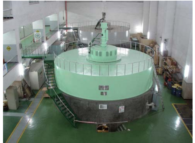
Chuncheon Hydroelectric Power Station, Korea
