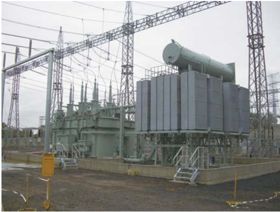
132 kV phase-shifting transformer at Armidale Substation
