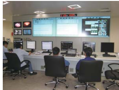
DCS operator station and large screen system
