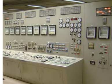
Previous plant control board
