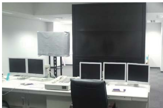
500 kV 変電所の制御室 Control room for 500 kV substation of The Tokyo Electric Power Co., Inc.
