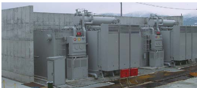
据付工事中の150 MVA主要変圧器 Installation of 150 MVA main transformer for Kurobe Substation of Hokuriku Electric Power Company
