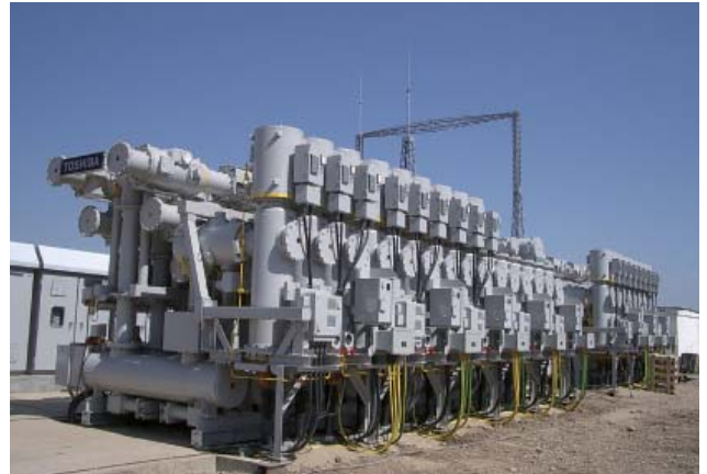
245 kV GIS at Romania Brazi Vest Substation
