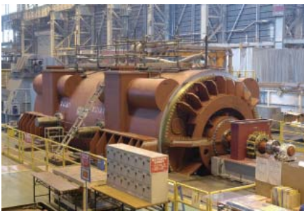
2P-60 Hz-1000 MW generator under performance test
