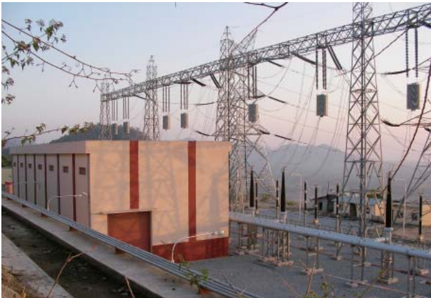
Overview of 400 kV substation
