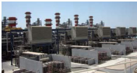
New power units of the Umm Al Nar Independent Water and Power Project
