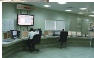
Central control room
