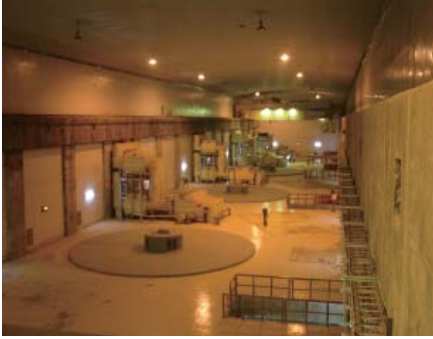
Overview of Purulia Pumped Storage Power Station
