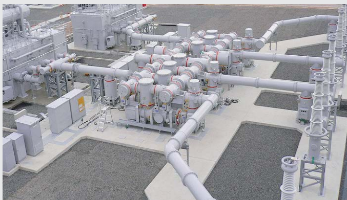
▲ 中部電力（株）亀山変電所向け300 kVガス絶縁開閉装置 300 kV gas-insulated switchgear for Kameyama Substation of Chubu Electric Power Co., Inc.
