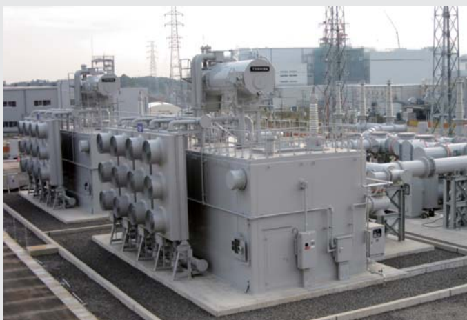
▲ 中部電力（株）亀山変電所向け275 kV-250 MVA変圧器 275 kV - 250 MVA transformer for Kameyama Substation of Chubu Electric Power Co., Inc.
