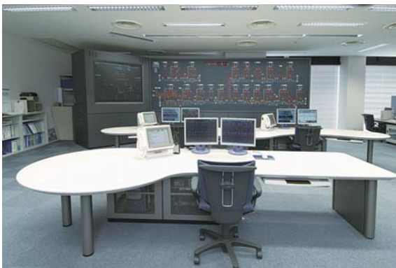
京王電鉄(株)向け 電力管理システム Supervisory control and data acquisition (SCADA) system for power supply systems of Keio Corporation
