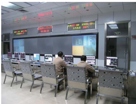
邢台発電所10、11号機中央監視制御室 Central control room of Xingtai Power Station Units No.10 and 11, China
