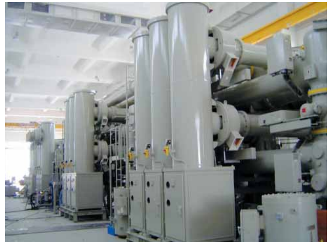
Site test of 400 kV gas-insulated switchgear (GIS) at Abu Dhabi Umm Al Nar IWPP Substation
