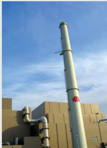
▲中部電力(株) 浜岡5号機 Hamaoka Nuclear Power Station Unit No.5 of Chubu Electric Power Co., Inc.
