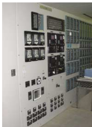
DⅢ-S形リレーに更新したBTG (Boiler, Turbine, Generator) 盤裏面の外観 Back appearance of boiler, turbine, and generator boards to be replaced by DⅢ-S type relay
