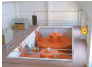
The Batuteqi Power Station (2×14.8 MW, August 2002), Indonesia
