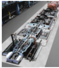
View of installed steam turbine and generator
