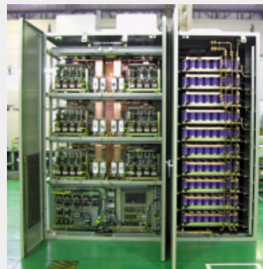
STATCOM (SVCS™) unit with application of IEGT
