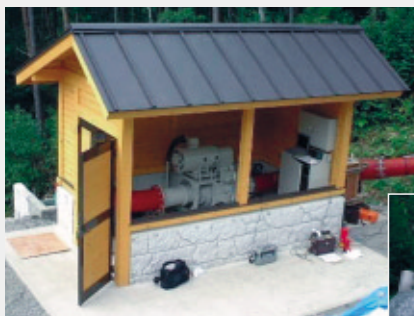
建設中のHydro-e KIDS™ S型 Hydro-e KIDS™ type S system under construction
