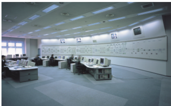
運転指令室概観 Overview of operation control room
