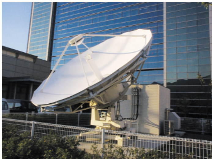
Ka帯地球局 Ka-band earth station
