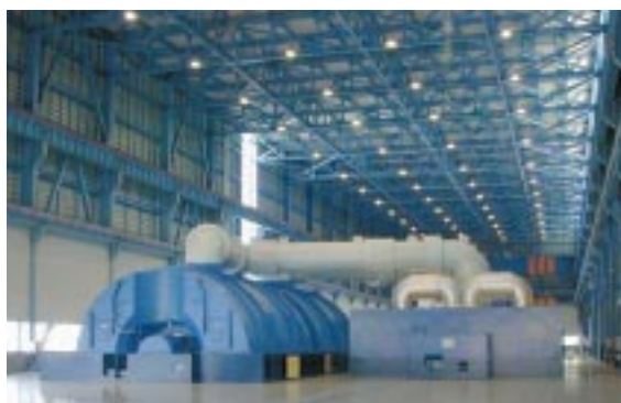
蒸気タービン外観 Appearance of steam turbine
