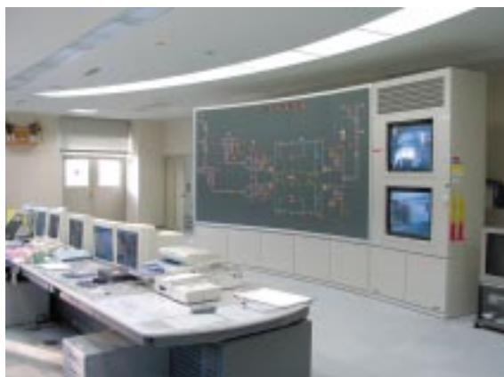
監視制御室 Control room at Anan Convert Station
