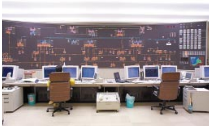
監視制御システム Supervisory control and data acquisition (SCADA) system at Fukui Regional Control Center
