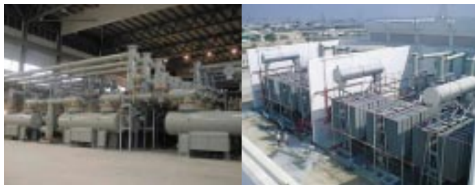
シンガポールTUAS向け400 kV変電所(左)とアブダビADPS向け400 kV変電所(右) 400 kV substations of TUAS, Singapore (left) and ADPS, Abu Dhabi (right)
