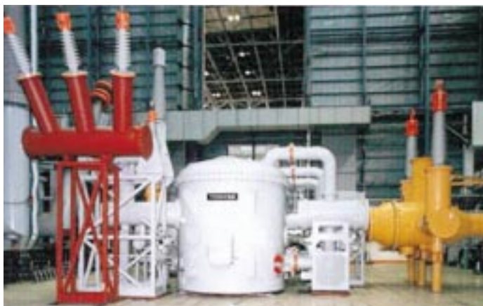
154 kV・200 MVAガス絶縁変圧器 154 kV-200 MVA gas-insulated transformer
