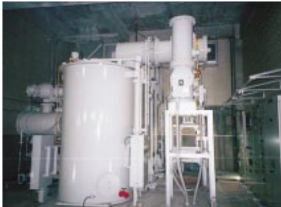
66 kV・60 MVAガス絶縁変圧器 66 kV-60 MVA gas-insulated transformer
