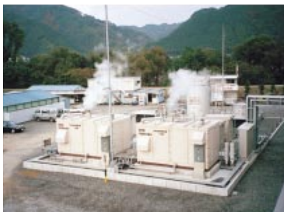
排メタノール燃料にて運転中のPC25™C (セイコーエプソン豊科事業所) PC25™C fuel cell power plants fueled with waste methanol from semiconductor factory
