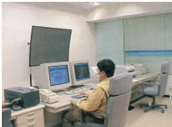
配電指令室 Control room of distribution automation system
