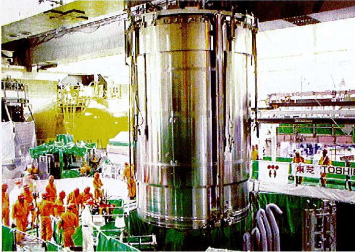
炉心シュラウドの原子炉内への吊込み Installation of core shroud into reactor pressure vessel
