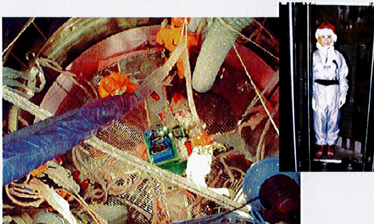
炉内化学除染および遮蔽体取付け後の原子炉内作業 Work in reactor pressure vessel after chemical decontamination and installation of shield
