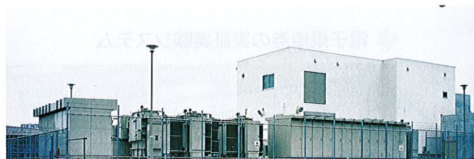
羽田変電所の外観 External view of Haneda Substation
