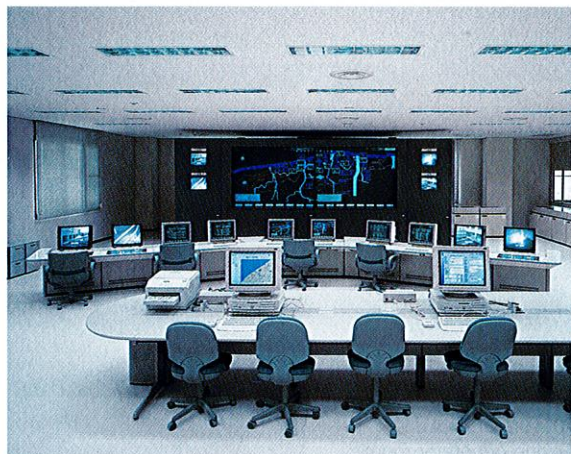
中央監視制御室 Central supervisory and control room
