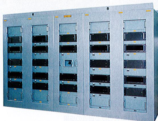
2F-1 DPRNM 盤 Digital power range neutron monitor(DPRNM)control panel for 2F-1 nuclear power station
