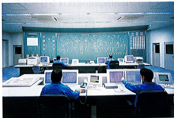
室蘭系統制御所の制御室 Operations room of Muroran Regional Control Center
