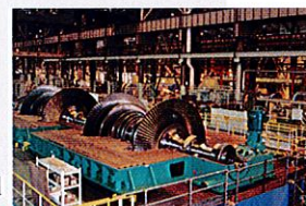
600MW turbine for Beilungang Power Station
