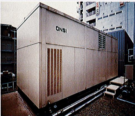
PC25 TM A 200kW fuel cell power plant in the Umeda Center Building
