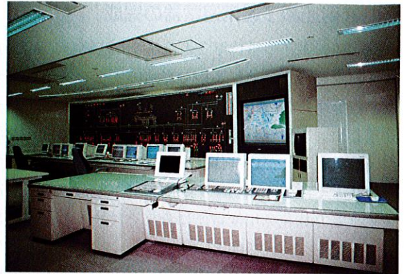
制御所指令室 Operating room of supervisory control and data acquisition (SCADA) system
