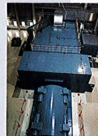
1,300°C-class, 154MW gas turbine, Unit No. 2 of the Chita Second Thermal Power Station
