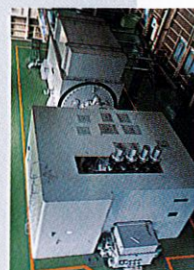
63.8MW steam turbine and generator, Unit No. 4 of the Osaka plant of Mitsui Toatsu Chemicals, Inc.
