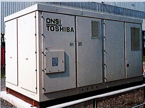
Commercial PC25 TM C 200kW fuel cell power plant
