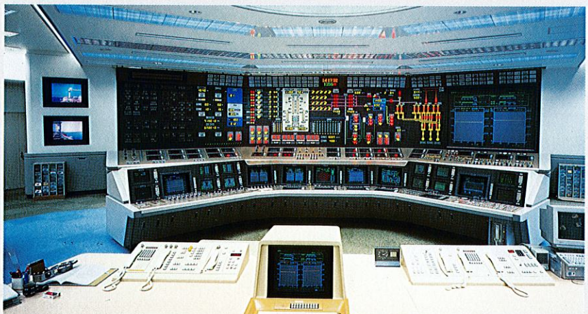
ABWRの中央制御盤 Main control panel of ABWR
