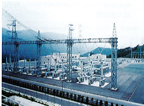
九州電力㈱脊振変電所 500 kV GIS・変圧器 500 kV equipment for Seburi Substation of Kyushu Electric Power Co., Inc.
