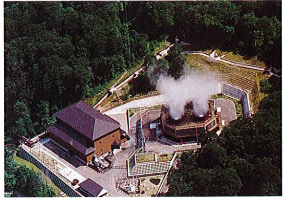
葛根田地熱2号機30 MW 蒸気タービン・発電機設備 30 MW steam turbine and generator at Kakkonda Geothermal Power Station No.2 Unit
