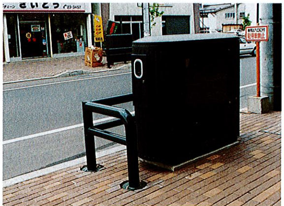
流雪溝水位監視盤 Supervisory control box of snow-floating disposal system
